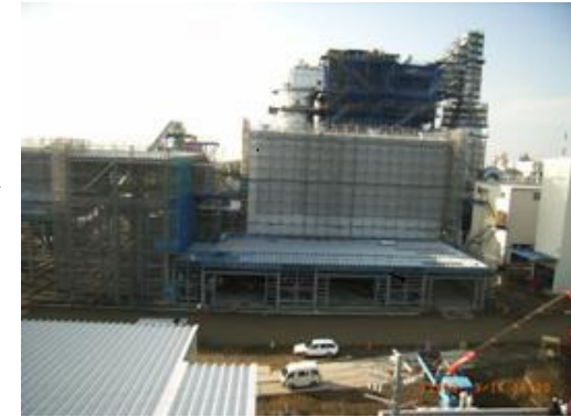
New incinerator at Eco-System Chiba
