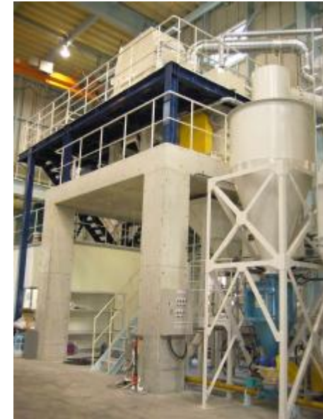
Strengthened sampling facility for platinum group metals
