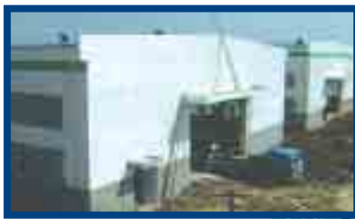
The first step in building a position in China: a precious metals recycling plant under construction (Suzhou, China)
