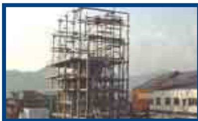
Automobile shredder residue (ASR) recycling facility under construction (Okayama City, Okayama Prefecture)
